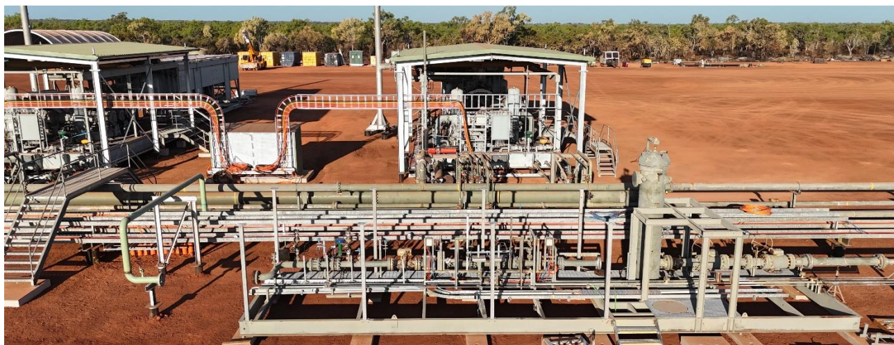
Carpentaria Gas Plant
