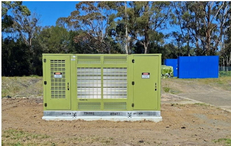
Figure 2: New TasNetworks substation installed at ALCORE Technology Centre
