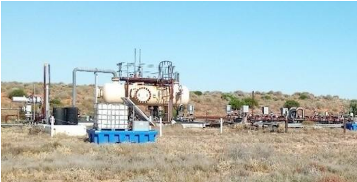
Figure 2: Vanessa Gas Field Facility
