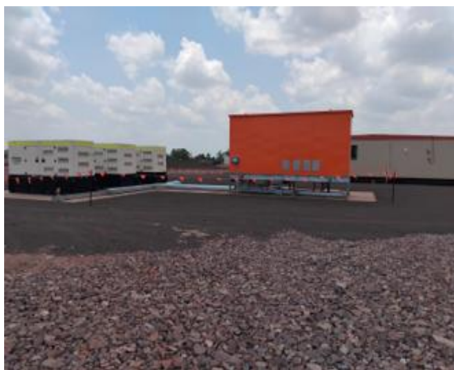
Figure 9: Camp Switchboard and Generators
