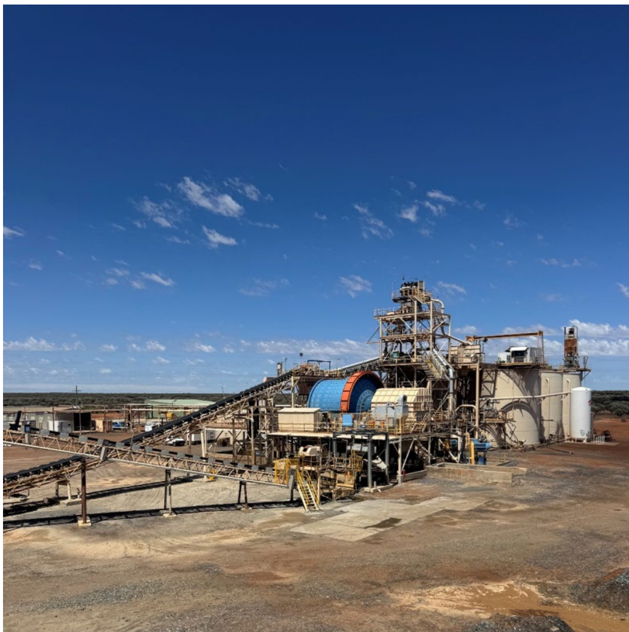
Figure 10: Kirkalocka process plant
