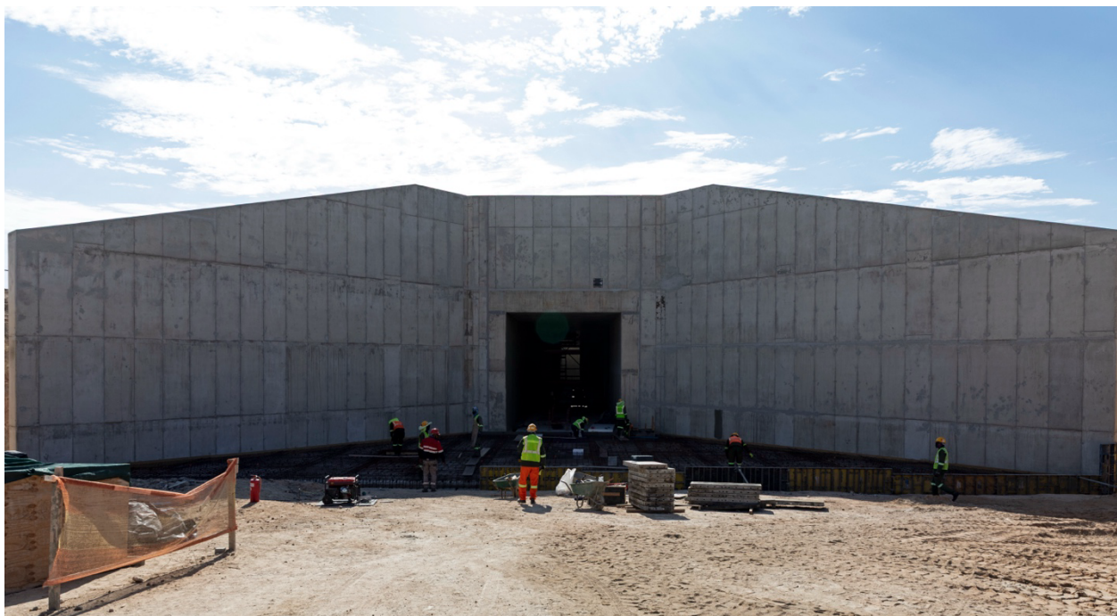
Figure 2. Conveyor exit at the coarse ore stockpile tunnel.
