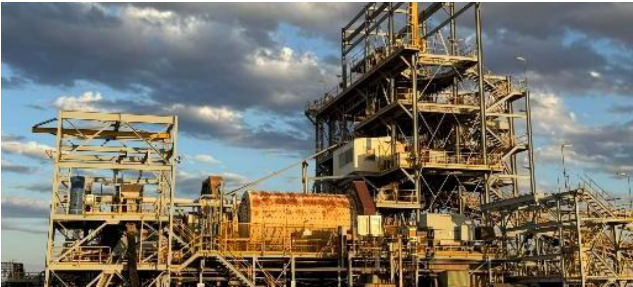
Concentrator Refurbishment Cost Estimation
