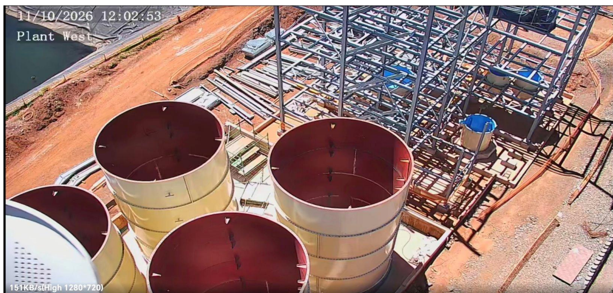
Figure 14: CIL tanks and elution buildings
