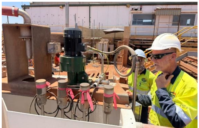
Bump testing of motors
