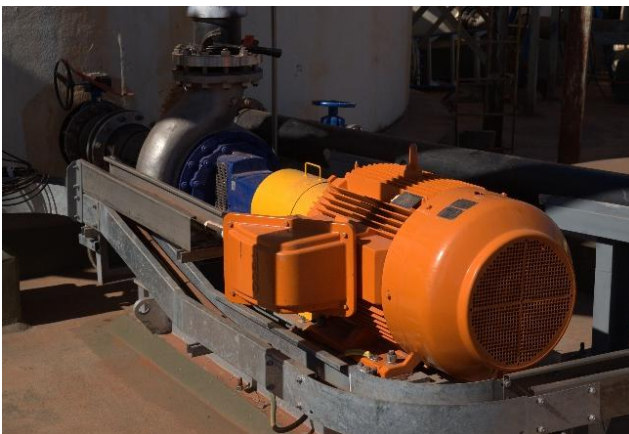
Pumps installed and commissioned
