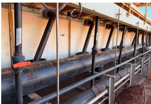
EW pipework installed
