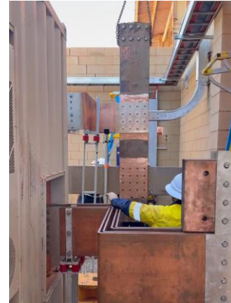
Rectifier busbar installed
