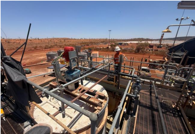
Mixer blade and rotor installed and bump tested
