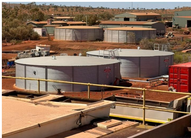
Firewater system installed
