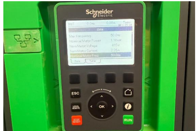
MCC energised with LV power
