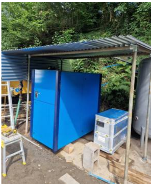
Above: New compressor unit installed
